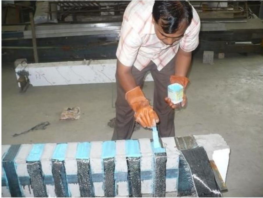
Fig. 53 Applying R&M Resin Matrix 20 on Concrete surface where CFRP was to be placed
