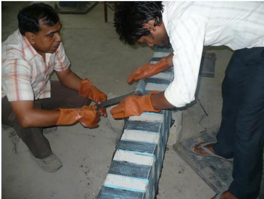
Fig. 54 Applying Roller on CFRP-Fabric to remove air bubbles between the CFRP and Concrete Surface
