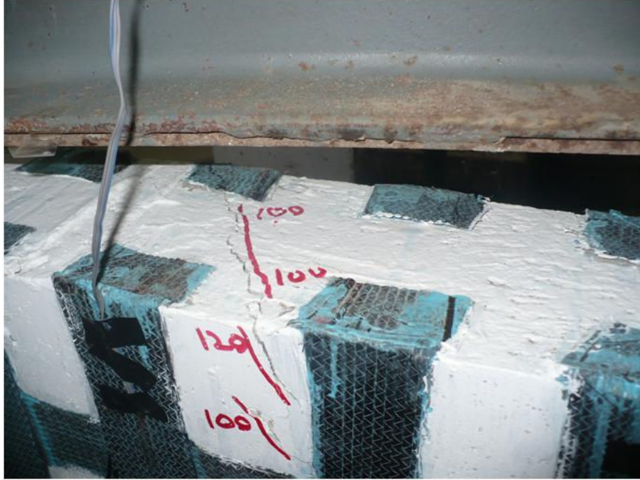
Fig. 82 Cracks formation at Average Torque 10.2 kNm (Total Load 120 kN) on Face F-1
