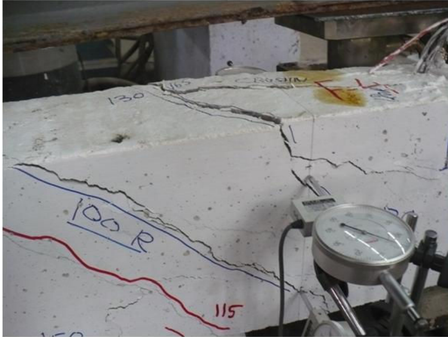
Fig. 71 Position of Cracks Total Load of 100 kN on Reversal of Loading at Face F-1
