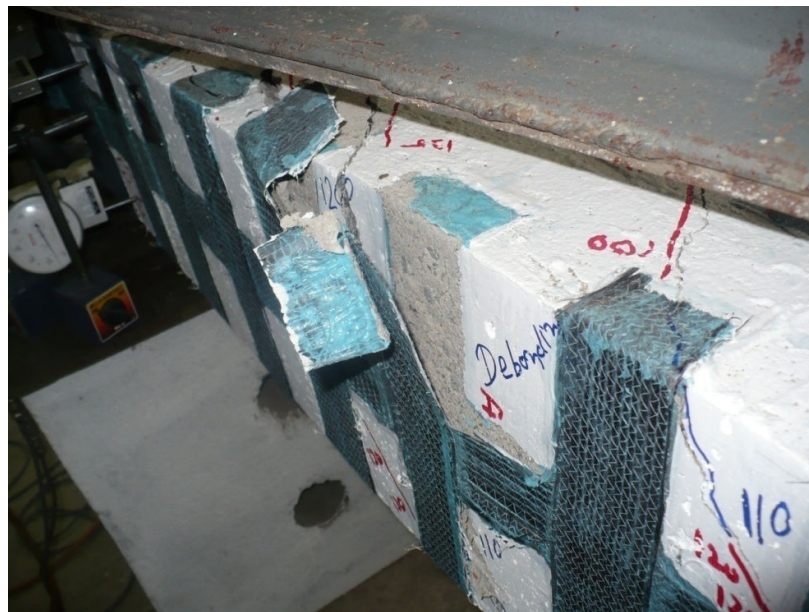
Fig. 86 Close View Debonding of Fabric Strips from Concrete
