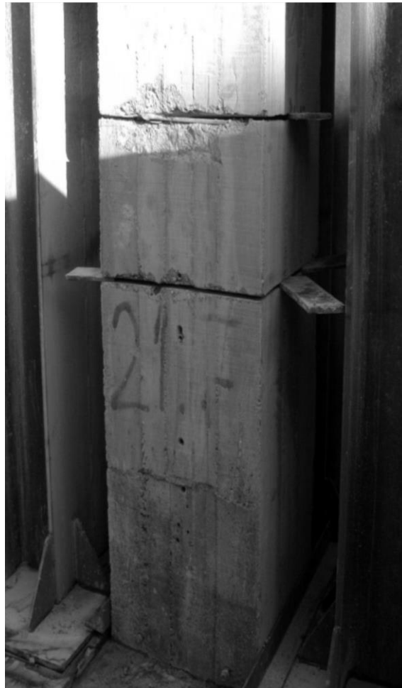
Fig 1.15: Saw cut through the concrete column
