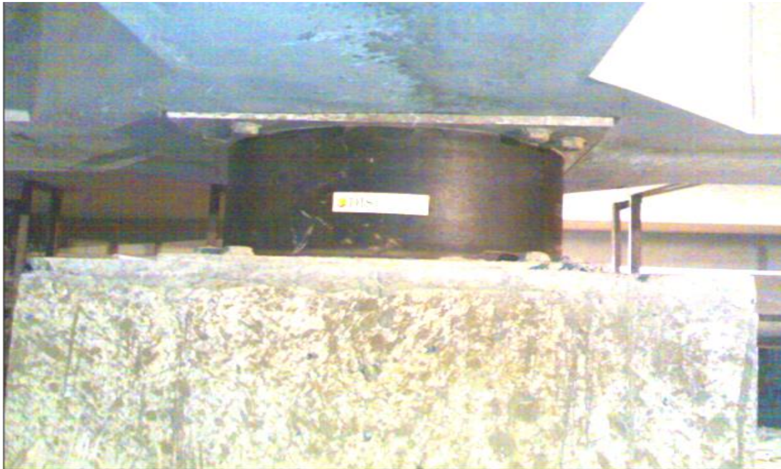
A View of “Lead Rubber Bearing “Installed in Basement at the Junction of Beam-Column in Base-Isolated Building At GTB Hospital Delhi.
