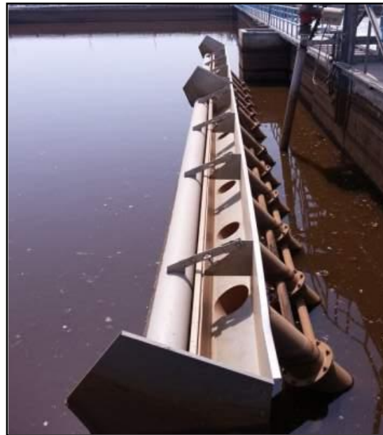
Figure 5.18: Fixed Type Decanter in SBR Tank
