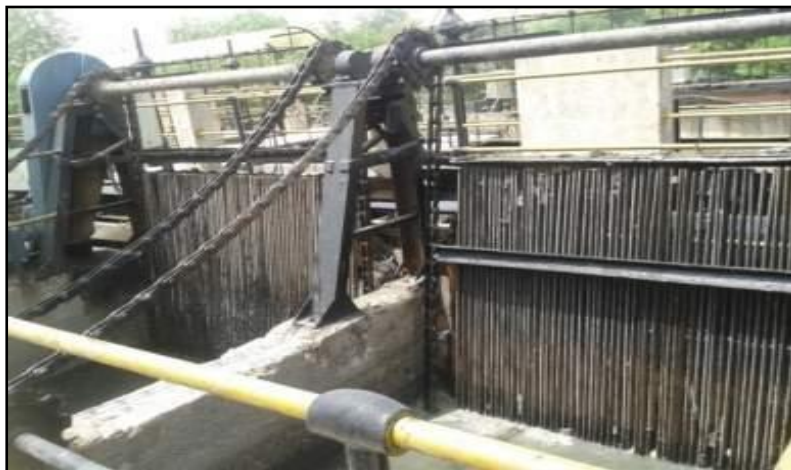
Figure 5.34: 20mm Mechanical Bar screens at ASP Plant inlet
