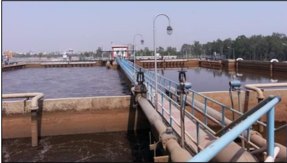
Figure 5.14: SBR Tanks installed at Indirapuram, Uttar Pradesh
