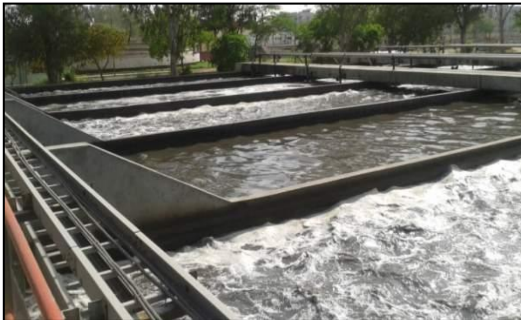
Figure 5.52: Oxidation Ditch installed at Phase-II, Rithala, Delhi
