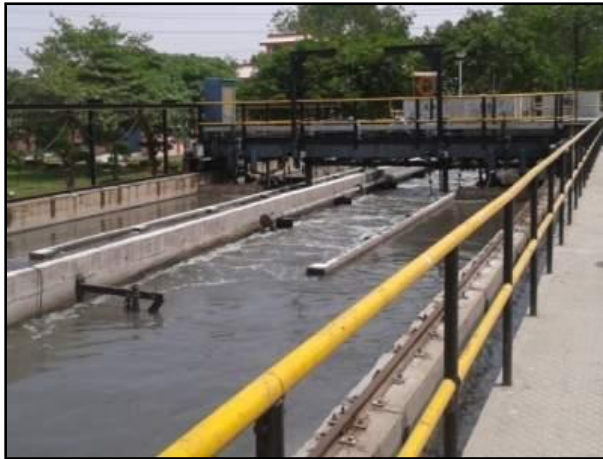
Figure 5.43: Grit Chamber Unit of ASP+BIOFOR Plant
