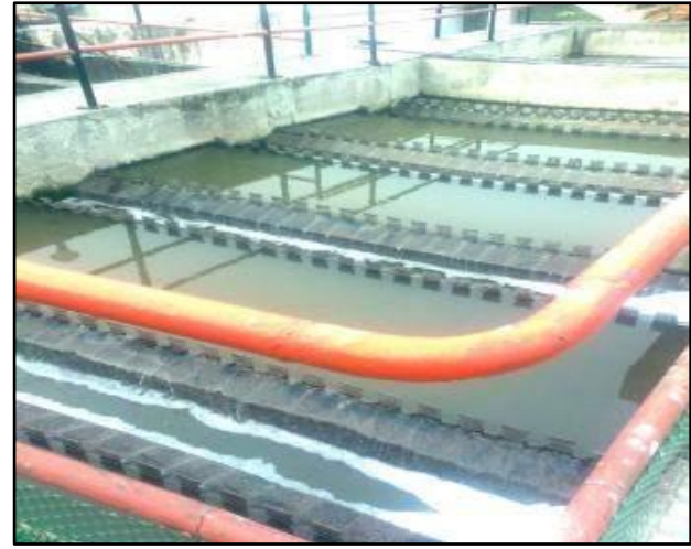
Figure 5.6: BIOFOR Stage – II Filtration
