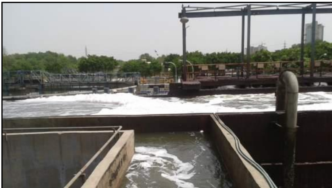
Figure 5.45: BIO Filtration Tanks after ASP installed at Phase-II, Rithala, Delhi
