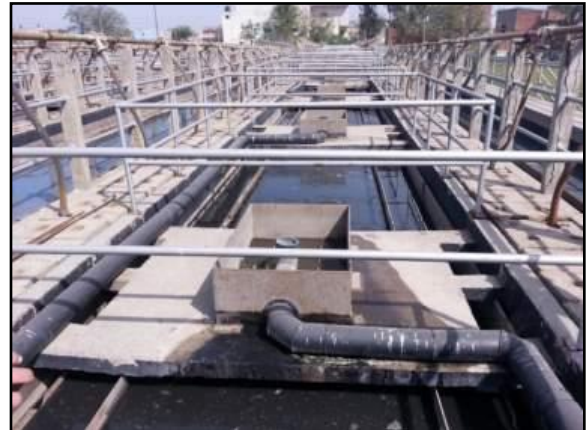
Figure 5.26: UASB Reactor installed at Dhanwapur, Gurgaon, Haryana
