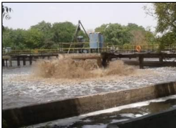
Figure 5.35: Aeration Tank of ASP Plant installed at Rithala, Delhi
