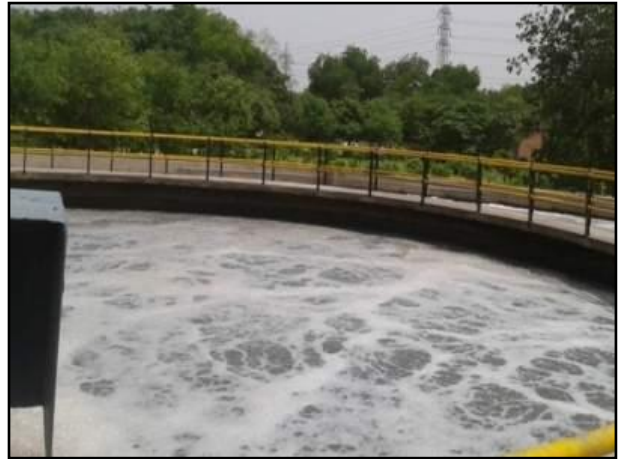
Figure 5.44: Aeration Tank of ASP+BIOFOR Plant
