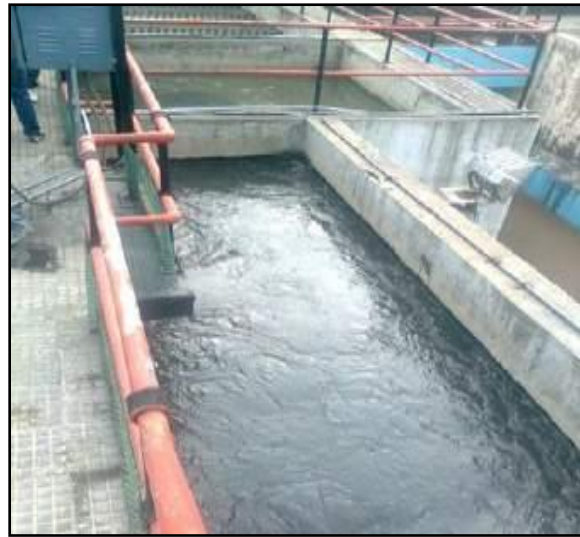
Figure 5.3: Grit and Grease removing unit
