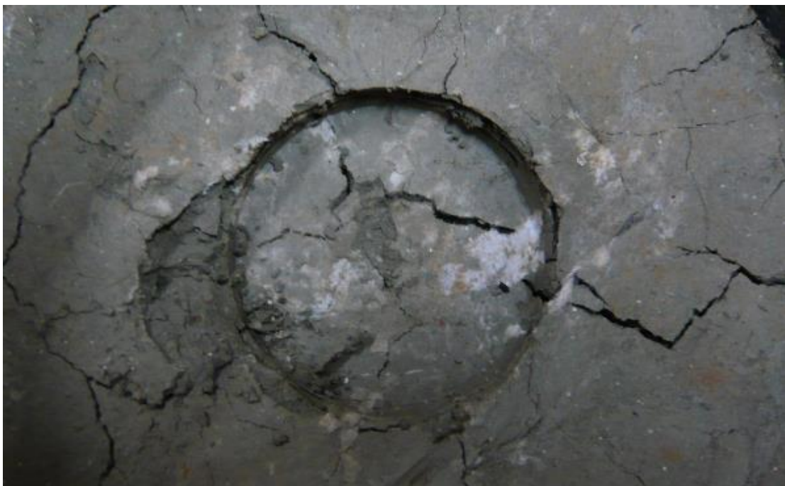
Figure 1.4 Cracks Developed in black cotton soil after drying
