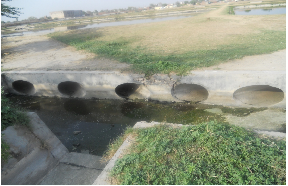
Fig 5.21B: Outlets of Trans-Yamuna STP, Mathura
