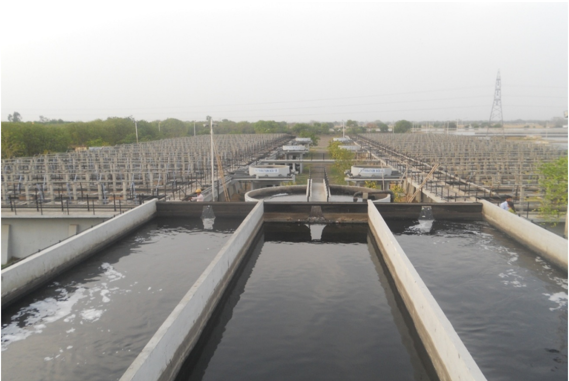
Fig 5.32: Grit Chamber and UASB at Dhandupura STP
