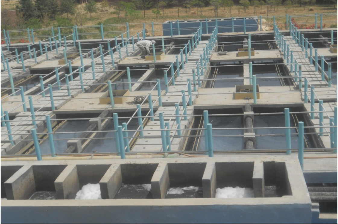
Fig 5.25: UASB at the Jaganpura STP.
