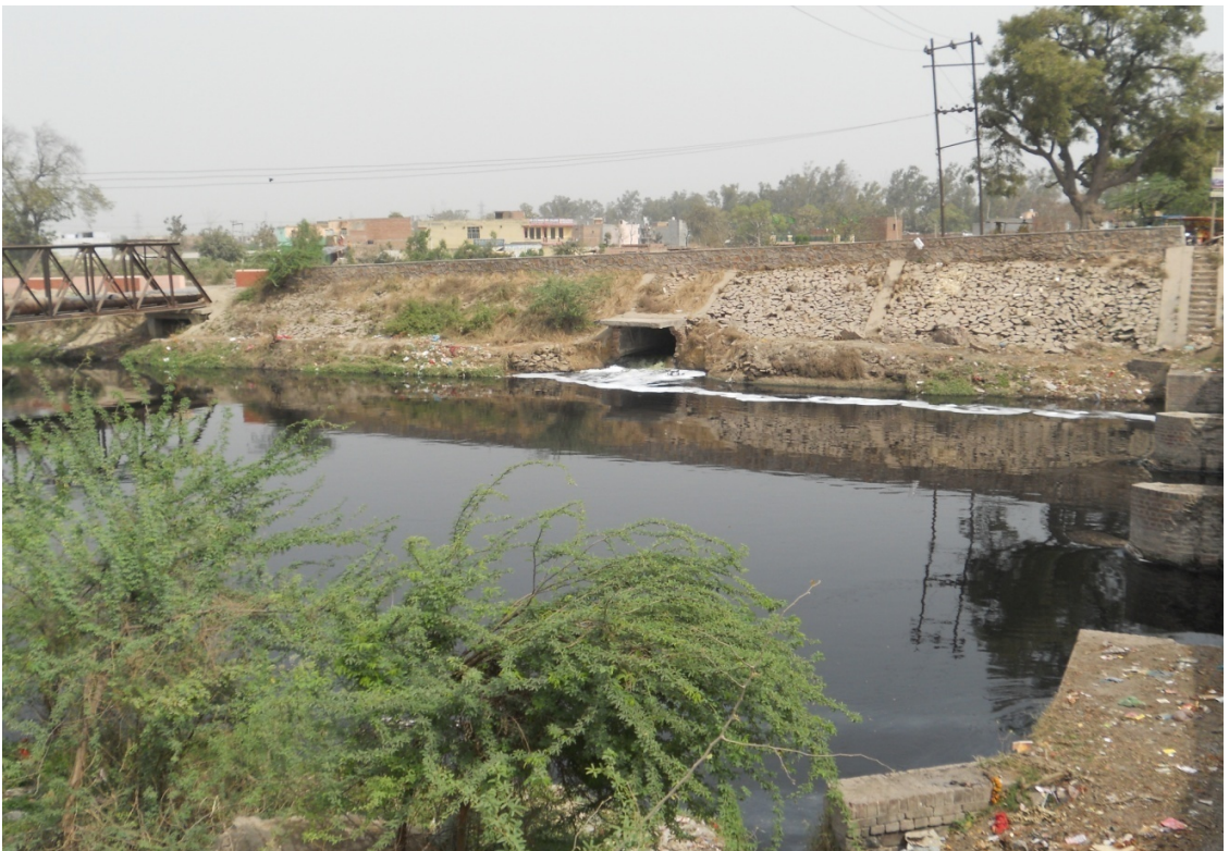
Fig 5.13: Agra Canal receiving the waste water from the STP outlet.
