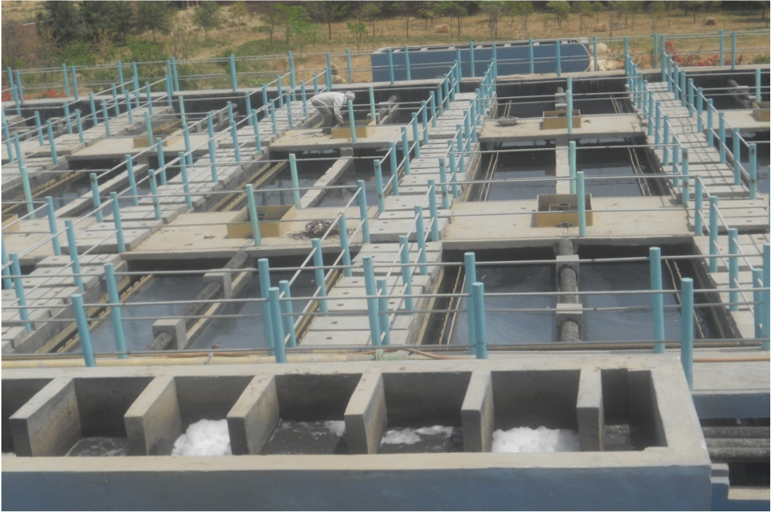
Fig 5.25: UASB at the Jaganpura STP.
