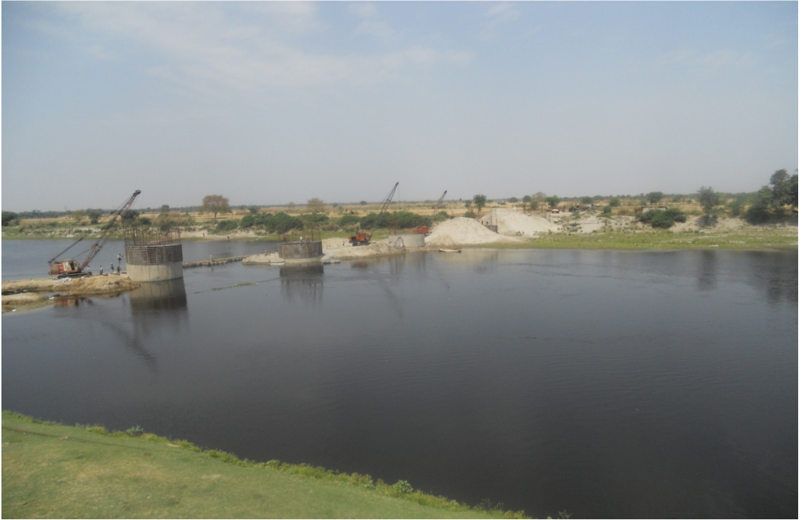
Fig 5.23: Water abstraction at Sikandara
