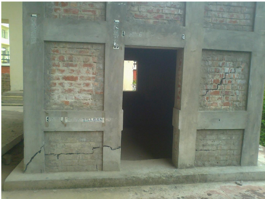
Fig.3.13: Performance of earthquake resistant brick masonry building due to shock
