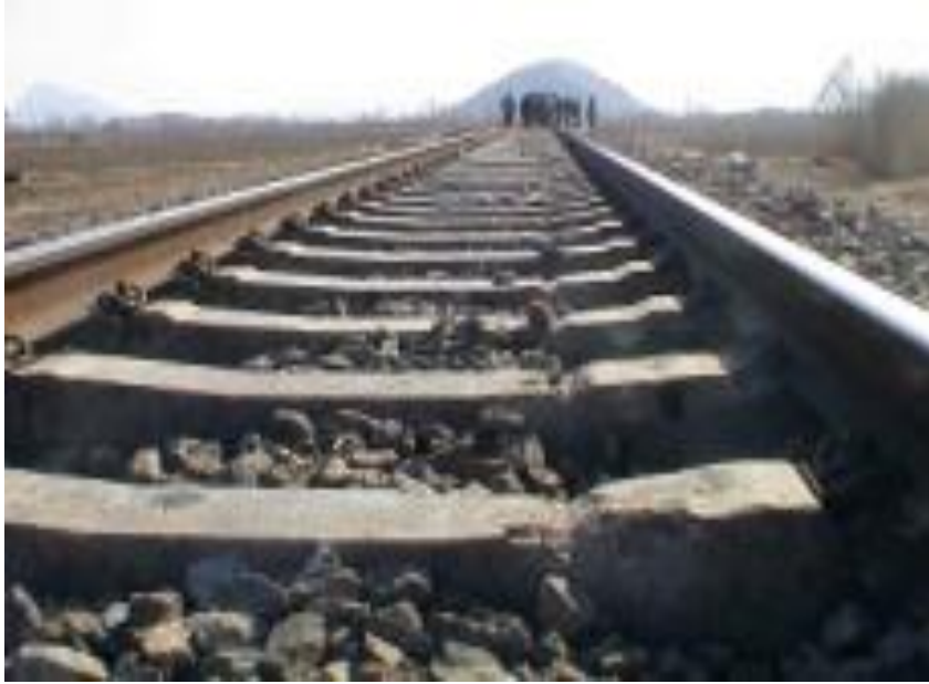
Figure 4.3 Sleeper breakage due to derailment
