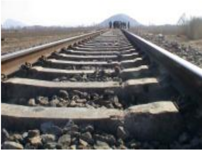
Figure 4.3 Sleeper breakage due to derailment
