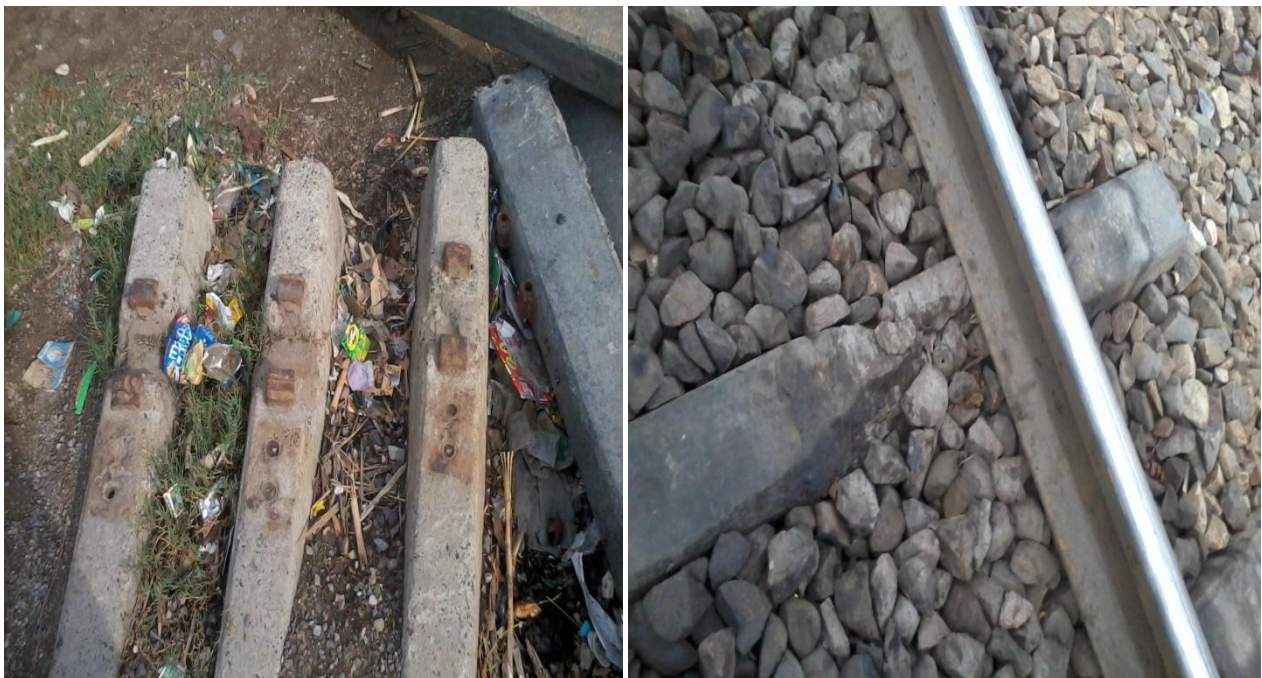
Fig4.5 – Defects during operation
