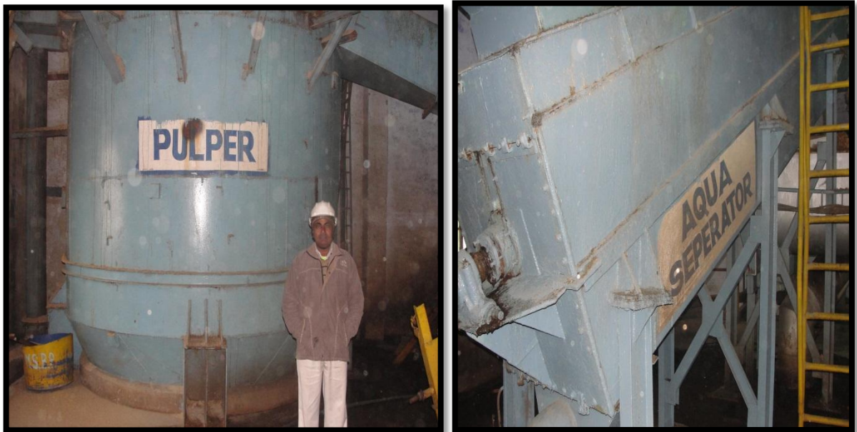
Figure 4.9: Wet Wash Pulping section (Pulper and Aqua Separator)
