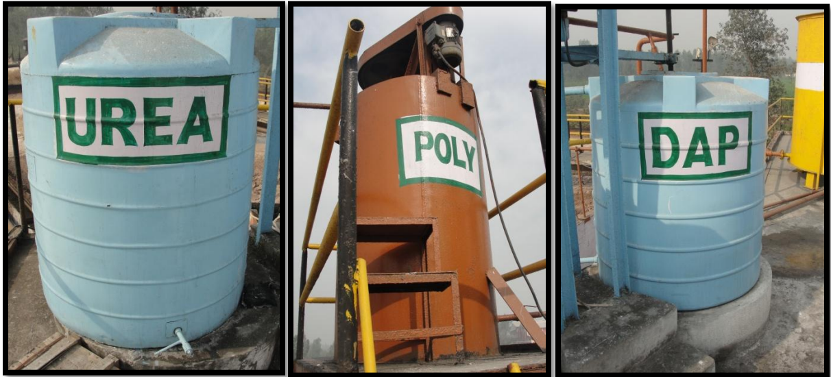
Figure 6.8: Chemicals Used in ETP Process (Naini Tissues Limited)
