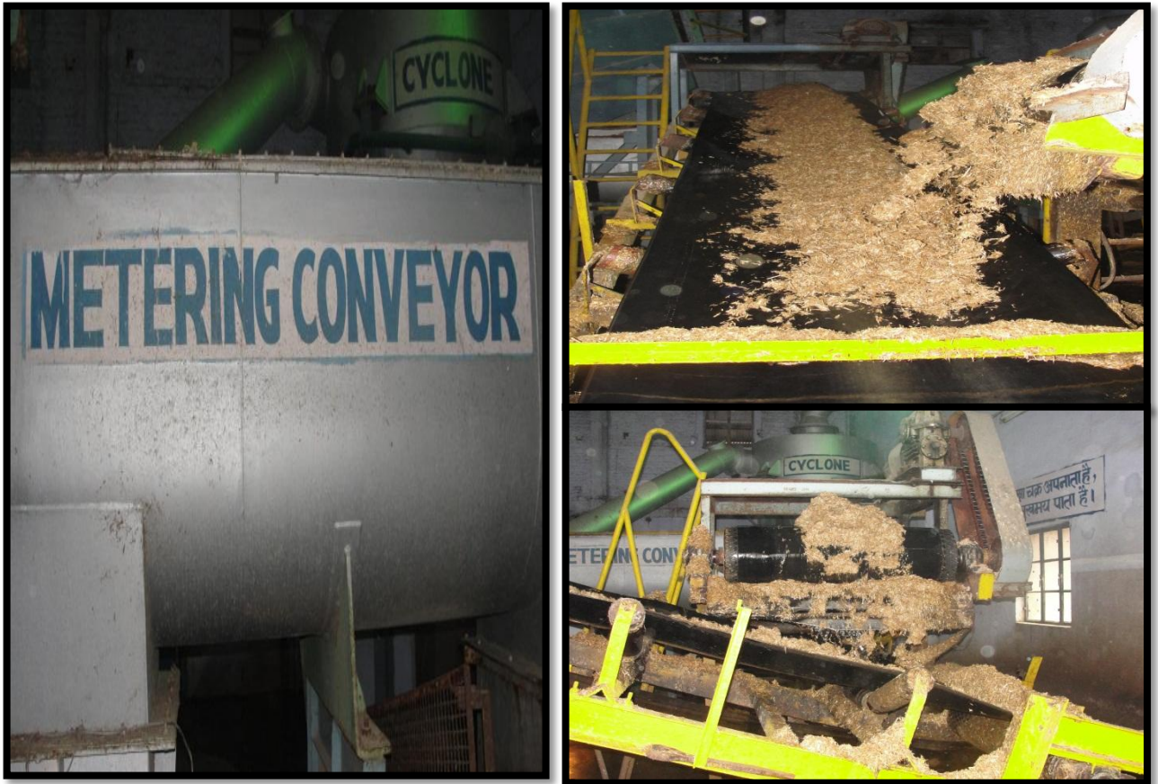
Figure 4.10: Metering Conveyor and Conveyor Belts
