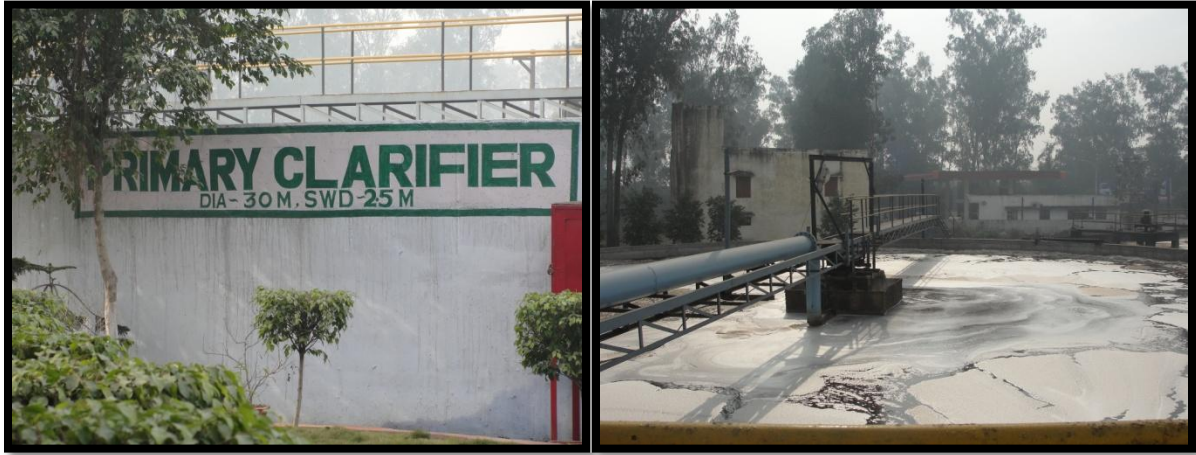
Figure 6.6: Primary Clarifier in ETP (Naini Tissues Limited)
