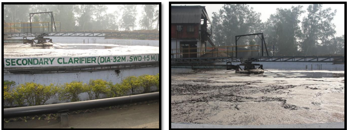
Figure 6.9: Secondary Clarifier in ETP (Naini Tissues Limited)
