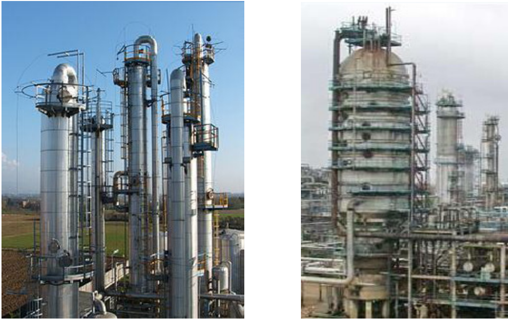
Fig. 4.4 A Typical Industrial Distillation Column
