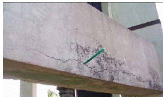
Figure 1.4: Crack in soffit concrete along the entire length of a staging
