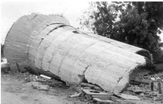
Figure 1.1: Collapse of water tank in Bhuj
