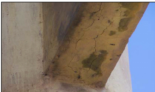
Figure 1.3: Crack in soffit concrete under side the staging beam of tank
