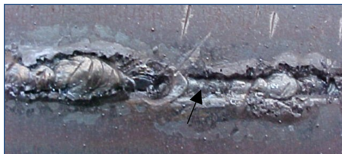
Figure 6.3d, Incomplete Penetration in Weld
